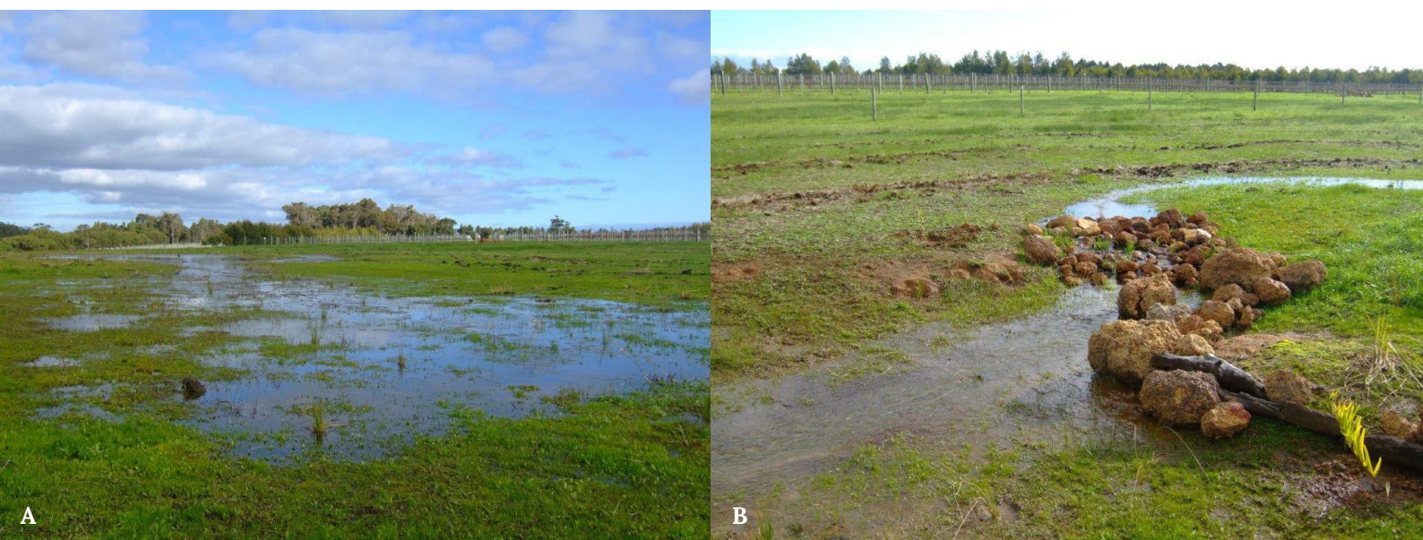
Figure 3. Rock pitching was used to decrease and direct the flow of winter catchment in watercourse B (refer to Figure 2); image A was taken prior to the rock pitches being installed, while image B highlights the extent to which the pitching has controlled water flow, preventing flooding of the paddock.
